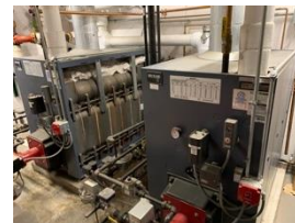
Boiler Room Alarms
